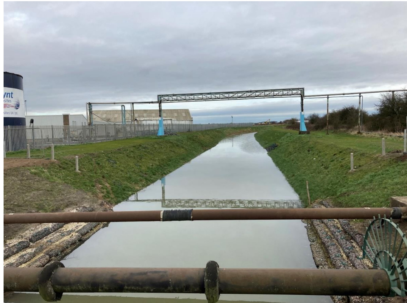
Figure 3: North Beck Drain looking downstream from Laporte Road towards the sea wall
